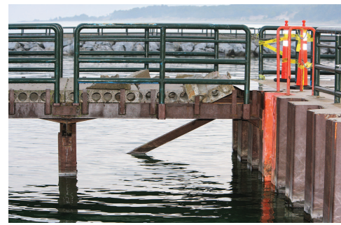
The first section of cement on the right (canal) side of the Charlevoix Lighthouse Pier is broken in pieces and marked with yellow caution tape to keep visitors off that half. The public is asked not to cross any yellow tape. PHOTOGRAPHY BY M. CHRIS LEESE
