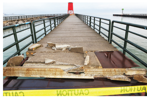
Dawn Tuesday morning reveals the concrete wreckage on the Pine River Canal side of the Charlevoix lighthouse pier, ribboned off with police tape to keep the public off that walkway until repairs can be made. PHOTOGRAPHY BY M. CHRIS LEESE
